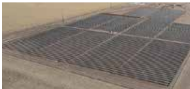
Johnson Corner Solar Project began commercial operation on April 7.
