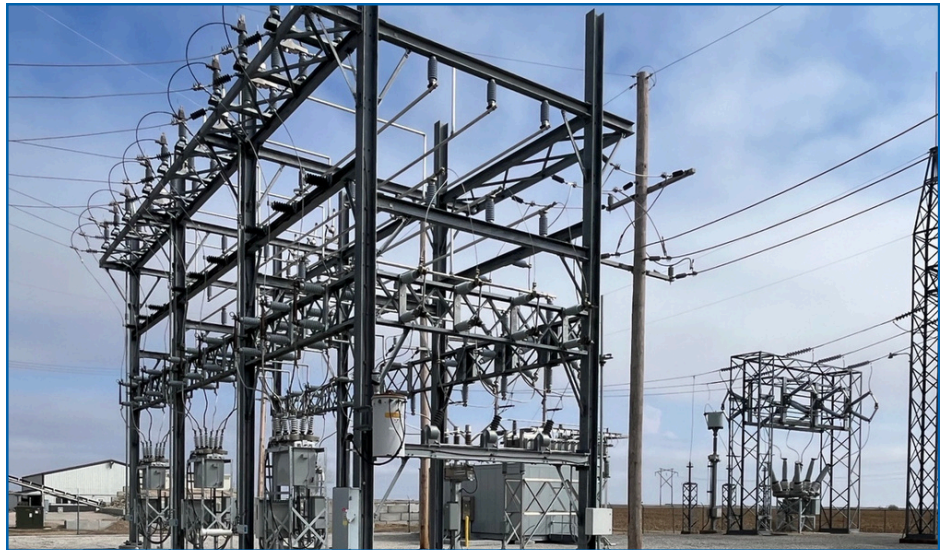
Upgraded Smith Center 115 kV substation equipment enables faster fault detection, improved system monitoring, and more reliable power delivery.
